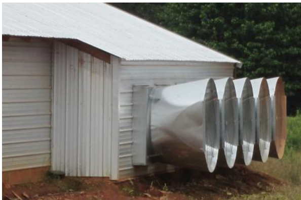
Tunnel fan light trap false wall installed in “dog house” or plenum in front of tunnel fans installed on the sides of the house.
