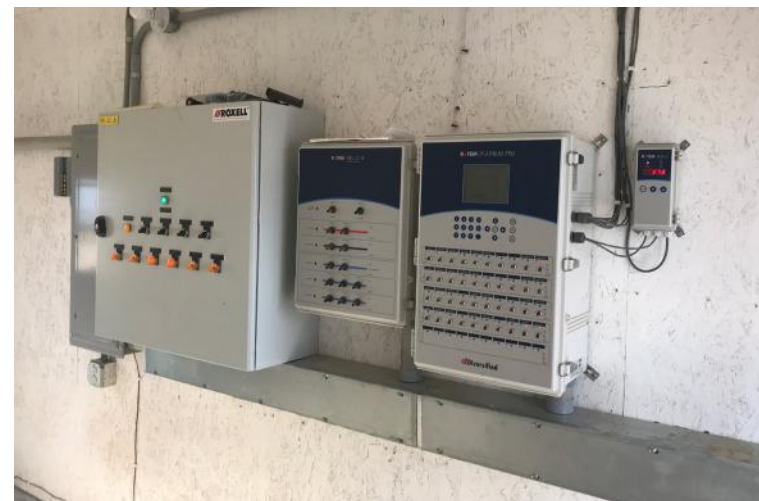
Verify that all systems are working correctly prior to chick placement.
