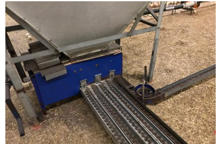
Run the feeding system and check that feed lines are level and secure.
